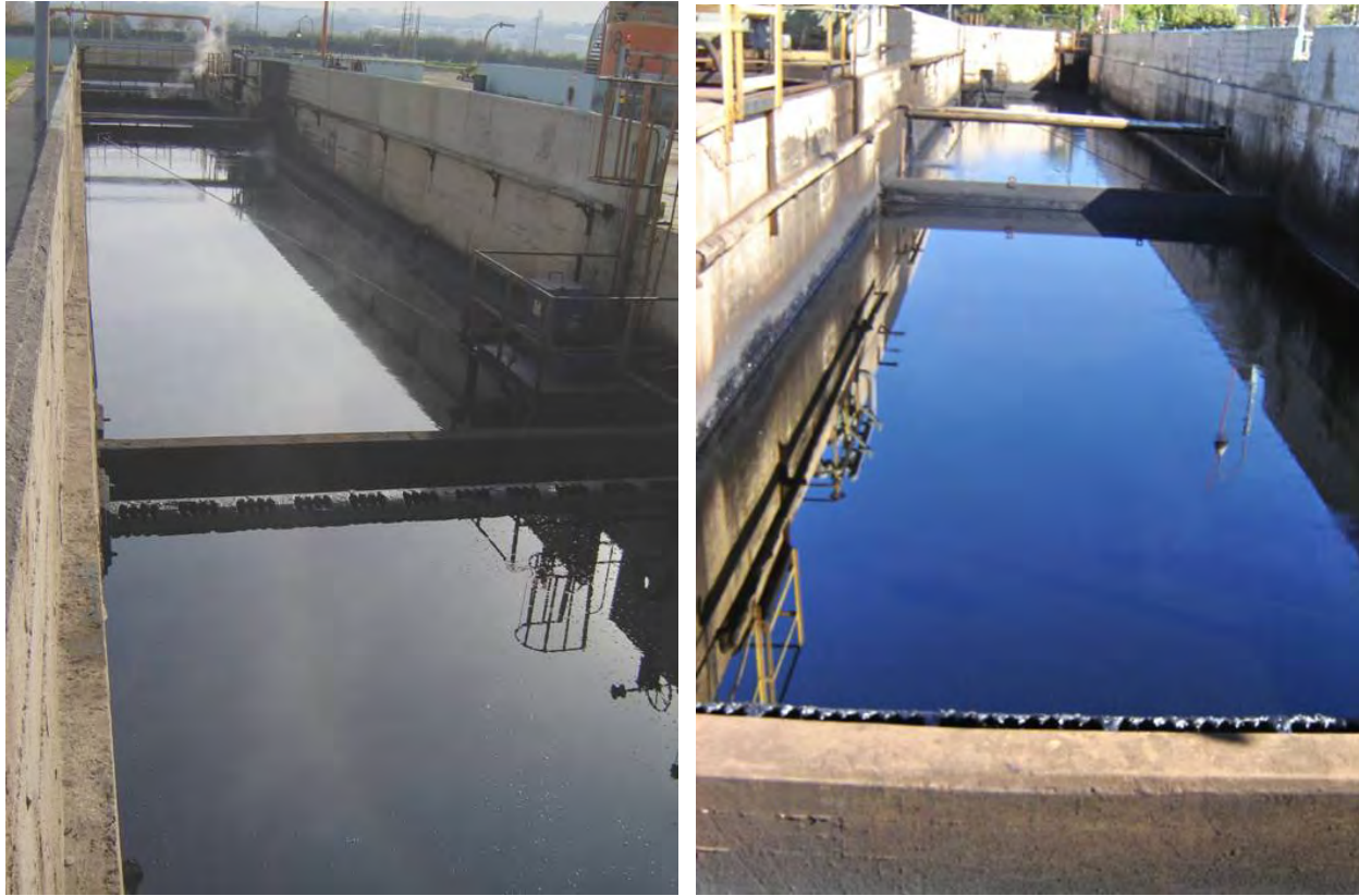
Figure 7: Typical API Separator, Left Flow Away from Camera, Right Flow towards Camera.
