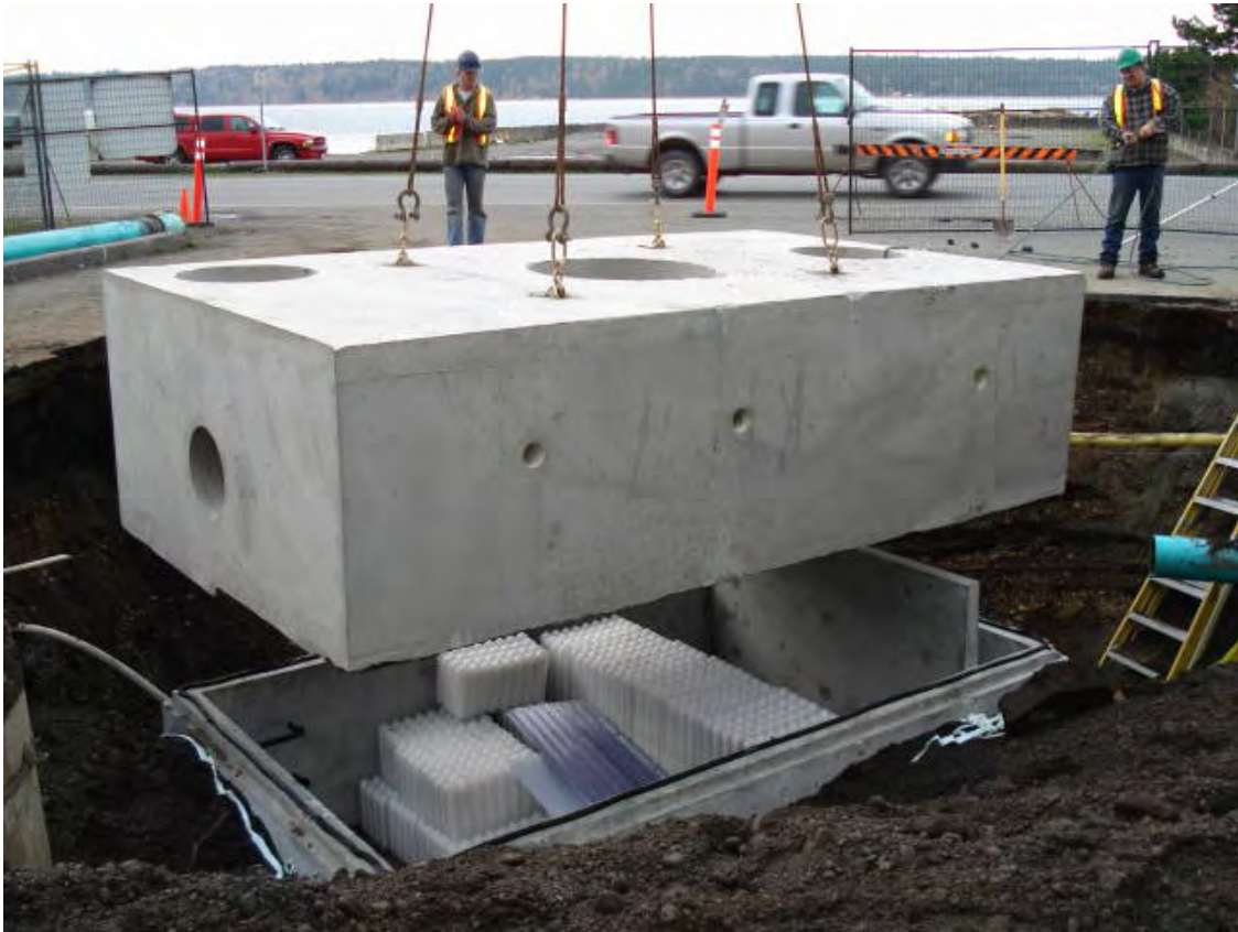
Figure 10: Typical Vault Utilizing Multiple Angle Plates (Photo courtesy Langley Concrete, Langley BC)
