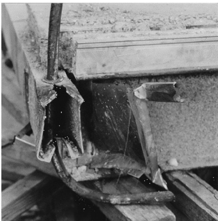
Figure 3 - Fourth Floor Walkway Box Beam Connection Failure
